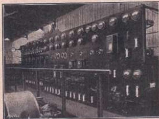
MAIN SWITCHBOARD, WEAVERHAM GENERATING STATION.
