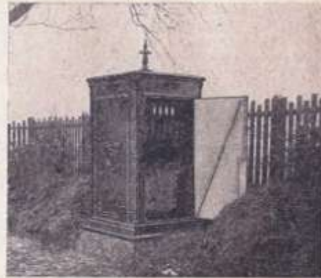
TRANSFORMER KIOSK AT SANDIWAY.
